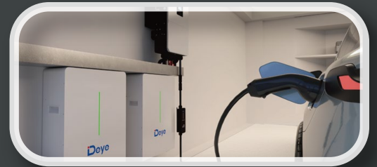
Smart EV Charger
